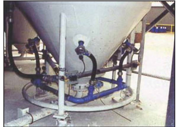
VA-12 AirSweep System mounted to the bottom of TiO 2 hopper.
