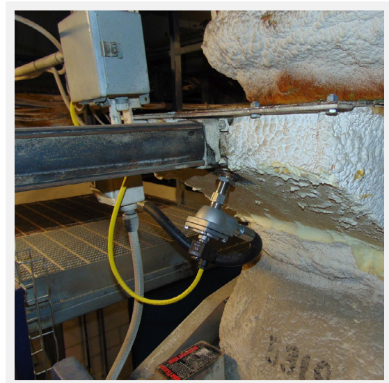
Strategically-positioned VA-12 units on dry-mix bin
